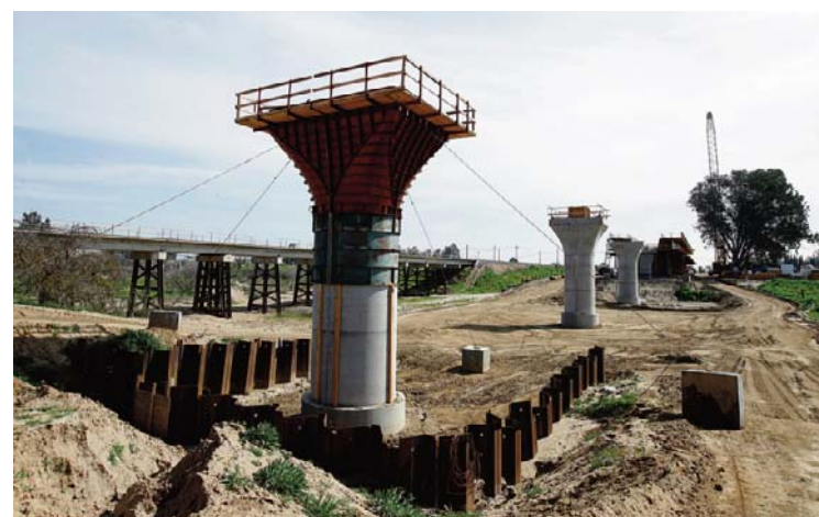
The supports for a 1,600-foot-viaduct to carry high-speed rail trains across the Fresno River are seen under construction near Madera, Calif. —AP
